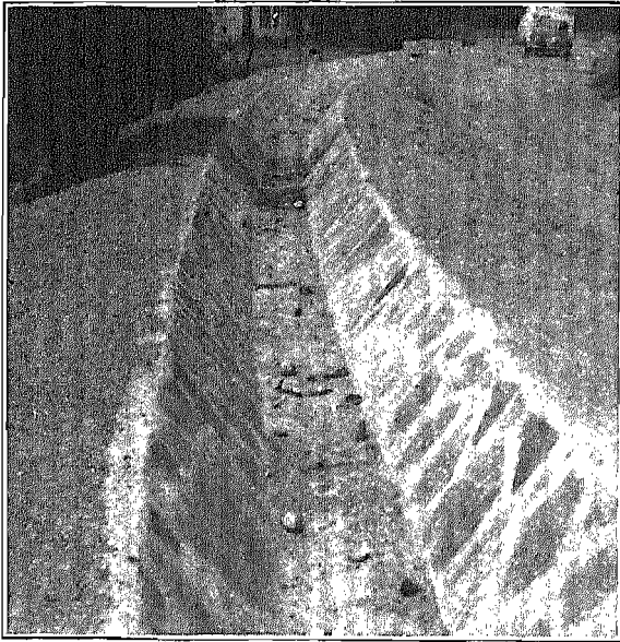
Fig. 38. A serviceable and attractive small Utah canal lined to solve the seepage, erosion, and weed problems. (Courtesy Work Projects Administration.)
