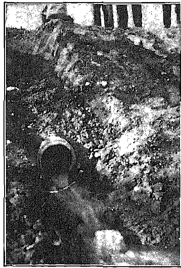
FIG. 149. The outlet-end of a 3600-ft, 8-in.-diameter concrete pipe drain immediately after installation during wintertime in Utah. (Photograph by J. R. Barker.)
