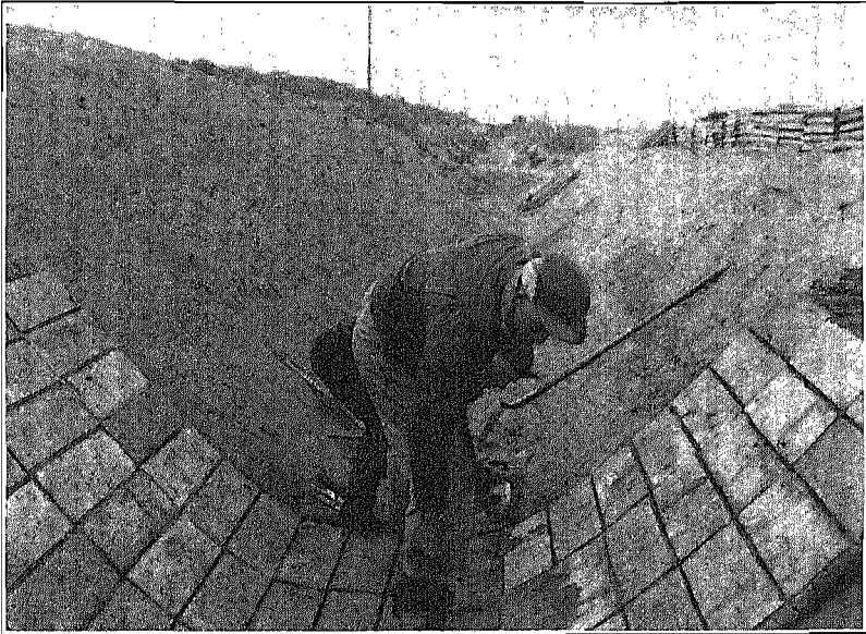
FIG. 37. Placing 8-in. by 24-in. precast concrete slabs with tongue and groove joints. Yakima Project, Washington, 1947. (Courtesy Bureau of Reclamation.)
