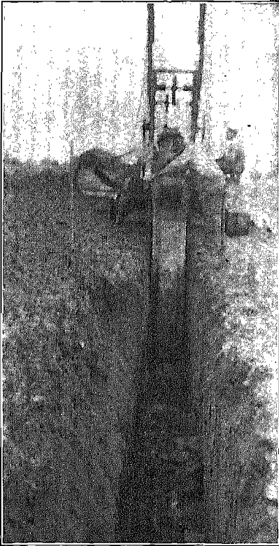
FIG. 148. Tractor-drawn excavator working in 6-ft-depth trench in sandy soil. The gravel over pipe joint can be seen near the cage. (Photograph by S. G. Margetts.)
