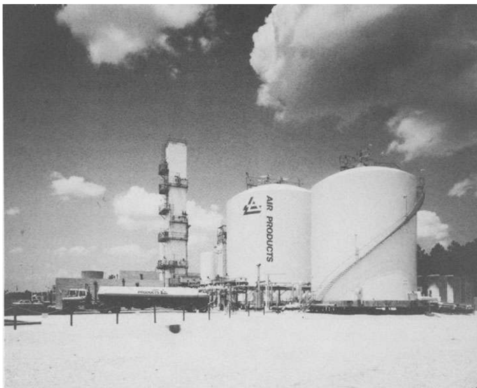
Fig. 13.1. Air separation plant including cryogenic storage tanks and cold box. (Courtesy Air Products and Chemicals, Inc.)
