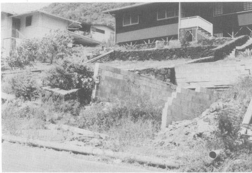
FIGURE 18.28 Structural failure caused by landslide on Vertisols produced by wet soil sliding downhill. Note that pipes are on top of the ground to prevent breaking caused by expansion and contraction of soil.
