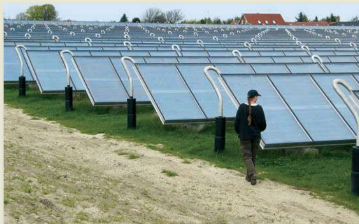
FIGURE 20.1 A 19,000 m 2 array of solar water heaters provides space heating for the town of Marstal on Ærø Island.
