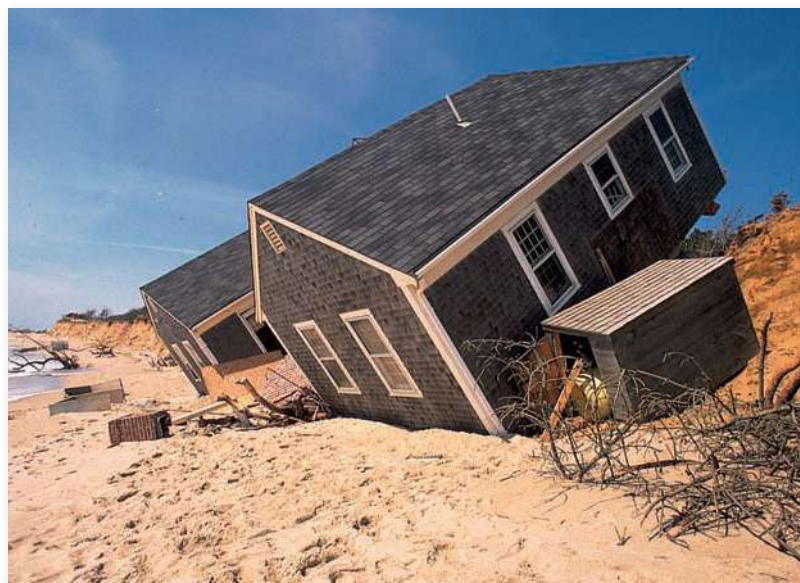
FIGURE 5.18 Winter storms have eroded the beach and undermined the foundations of homes on this barrier island. Breaking through protective dunes to build such houses damages sensitive plant communities and exposes the whole island to storm sand erosion. Coastal zone management attempts to limit development on fragile sites.
