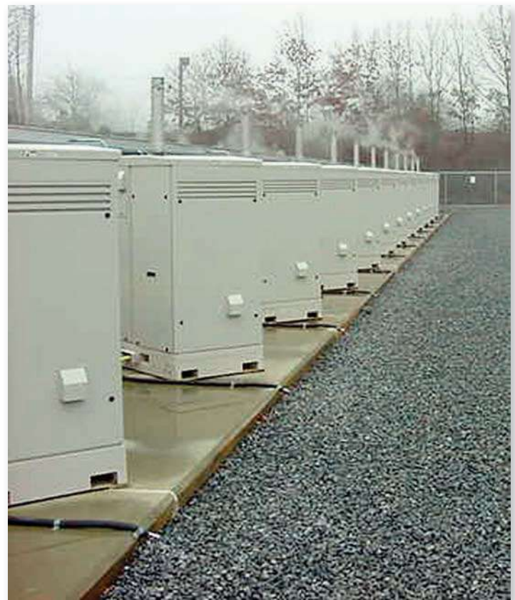
FIGURE 20.16 The Long Island Power Authority has installed 75 stationary fuel cells to provide reliable backup power.
