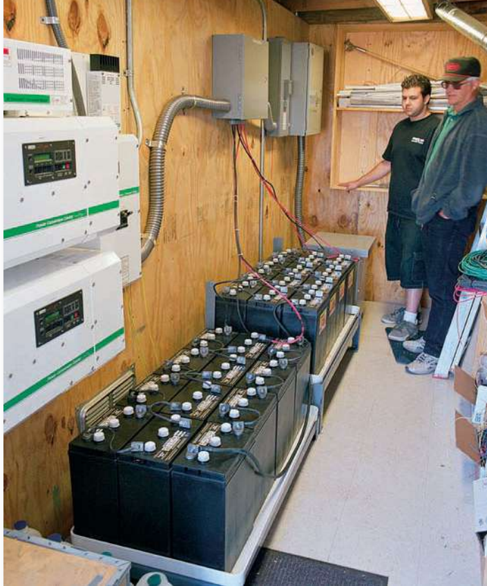
FIGURE 20.14 A large battery array, together with inverters and regulators, store photovoltaic energy on the Manzanita Indian Reservation in California.
