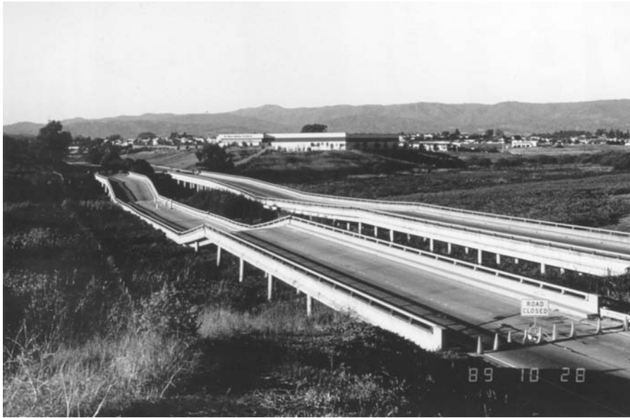
Figure 137 Highway 1 bridge destroyed by liquefaction of river deposits at Struve Slough during the October 17, 1989, Loma Prieta, California, earthquake.
