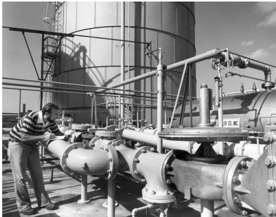
Figure 178 A facility designed to convert animal wastes into methane gas, Barton, Florida.
