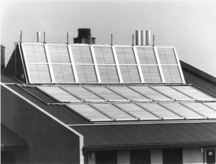
Figure 182 Solar panels on a laboratory at the University of California, Davis, California.
