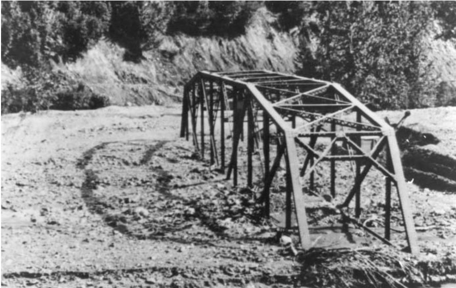
Figure 73 A bridge at Sheep Creek partially buried by debris from a glacier outburst flood, Copper River region, Alaska.
